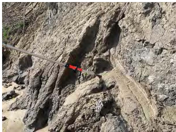
Picture 9: Soil seepage at base of bluff along beach.
