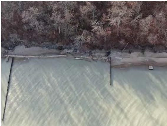
Picture 13: Aerial photo of deteriorating seawall on southern half of Section B.
