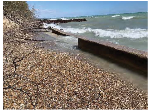
Figure 2.16 Scouring that is occurring behind the breached seawall.
