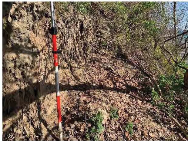
Figure 2.11 Slope failure at top of bluff on north end of Section C.
