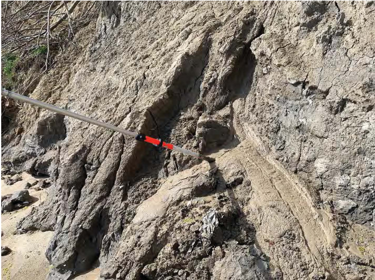
Figure 2.31 Liquifying soil seeping out the face of the bluff along the beach due to excessive soil saturation.
