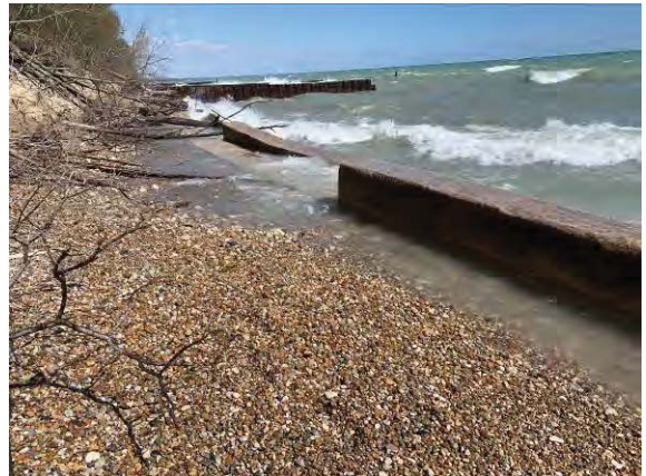
Picture 14: Washout occurring behind the seawall on the south of Section B.
