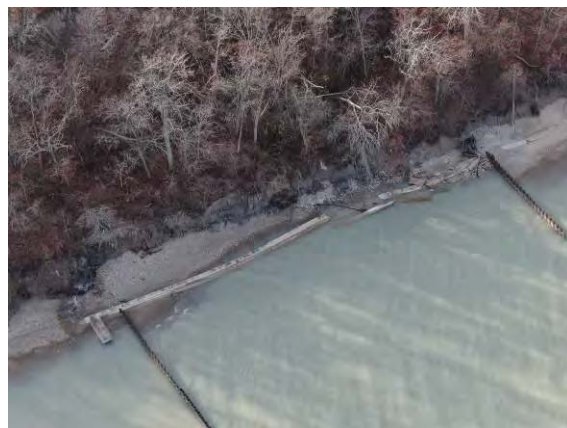
Picture 15: Slope failure behind seawall on south half of Section B.
