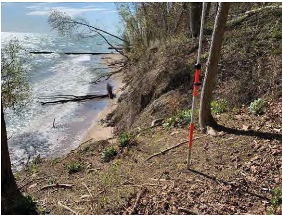
Picture 3: Major erosion and slope failure at beach.
