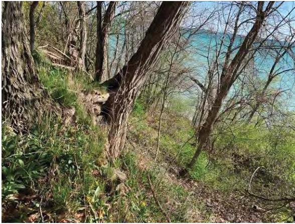
Picture 7: Tree in slope failure zone.
