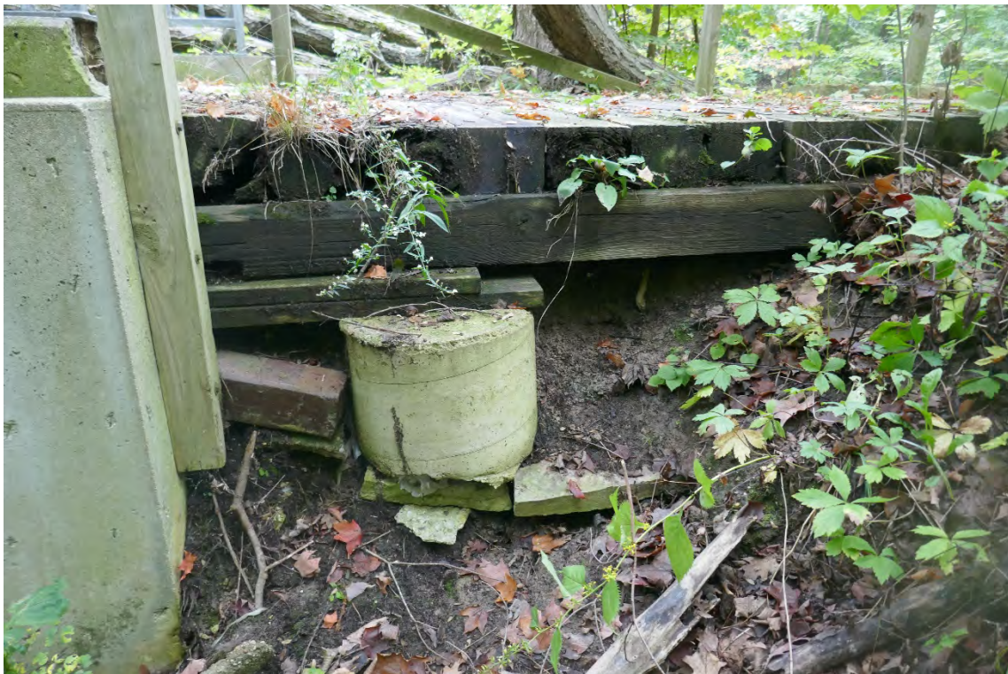
Erosion Under Path Adjacent to East Abutment
