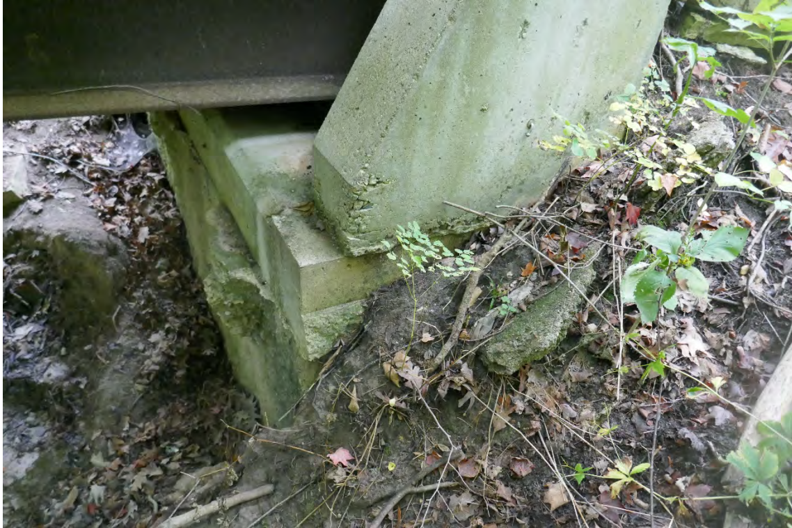
South Corner of East Abutment – Minor Erosion on Side
