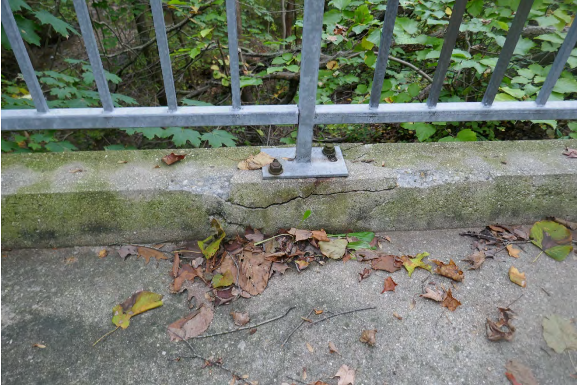
Typical Rail Post – Posts Were Previously Embedded, Now All Posts are Connected with Base Plates – Concrete Delaminating/Spalling at Several Posts
