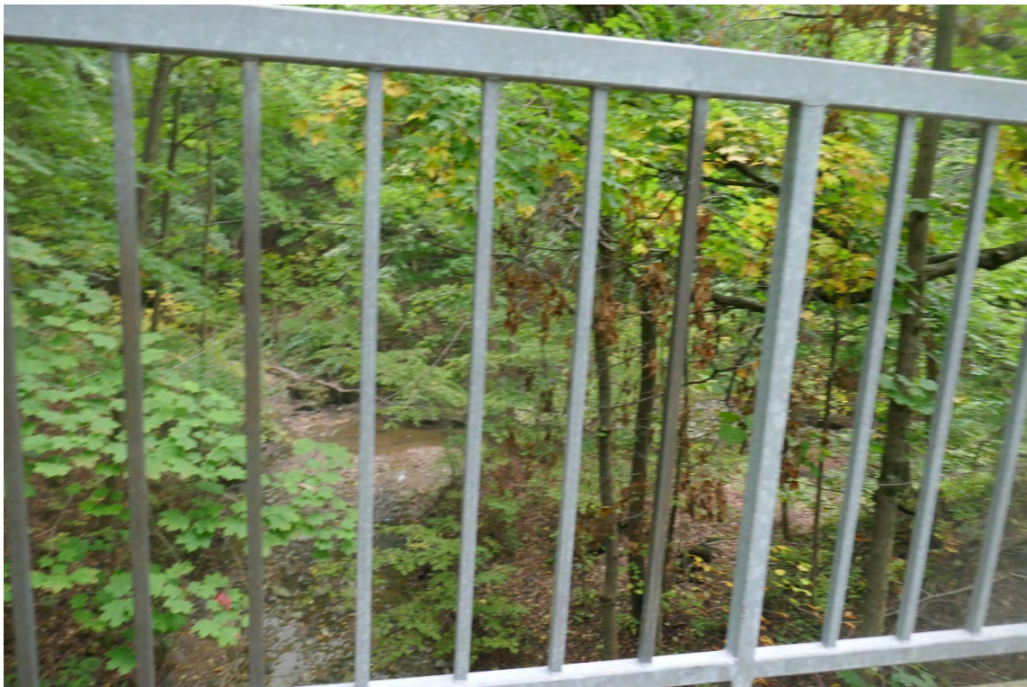
Typical Railing Condition
