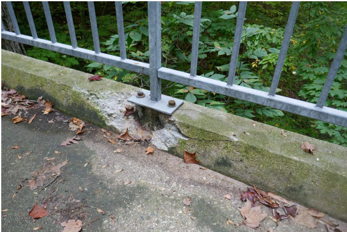
Concrete Spalling at Rail Post
