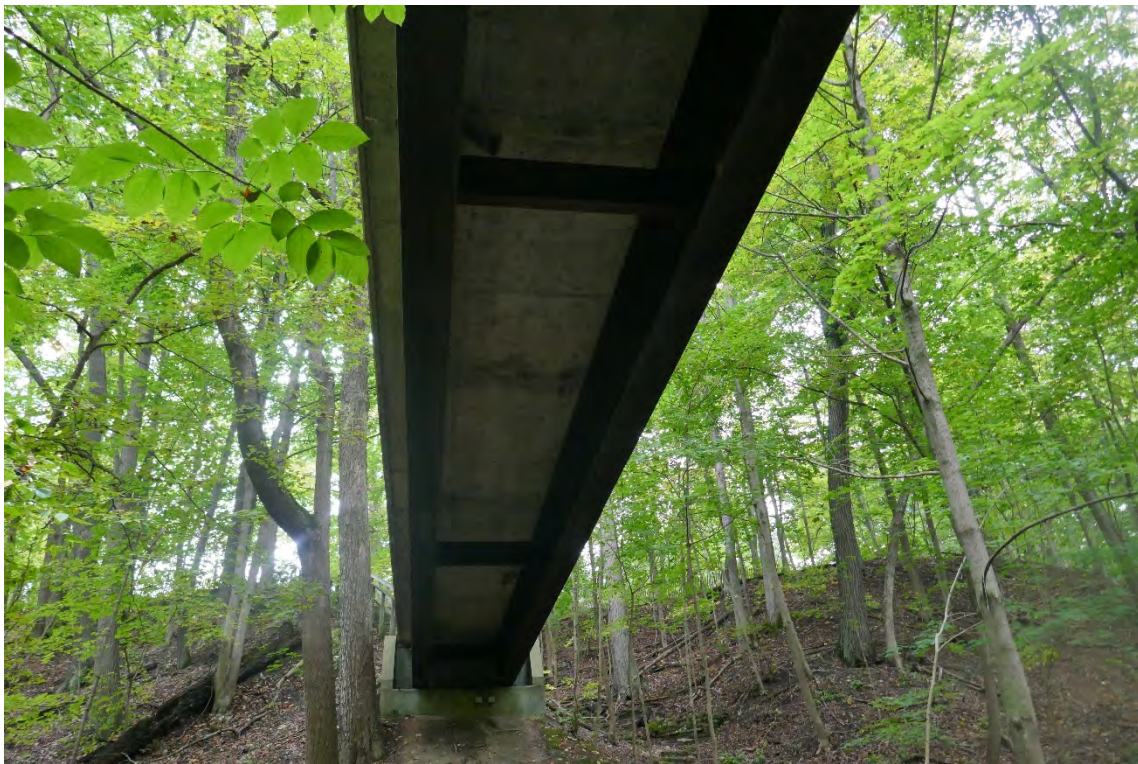
Typical Underside of Deck and Steel Superstructure (37" Weathering Steel Plate Girders) – Girders, Interior Diaphragms in Good Condition – No Issues Noted
