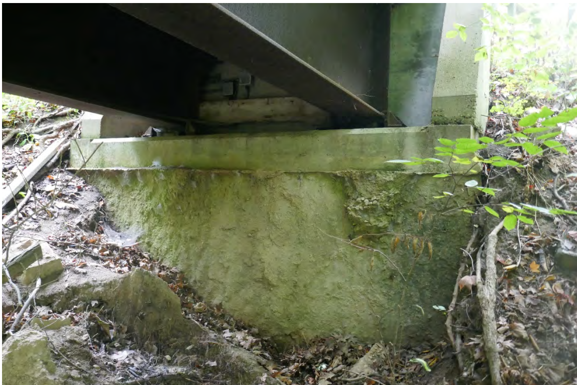
East Abutment – Minor Progression of Erosion at Abutment - Approximately 56" From the Ground to the Top of Beam Seat – Recommend Placing Embankment and Riprap Here
