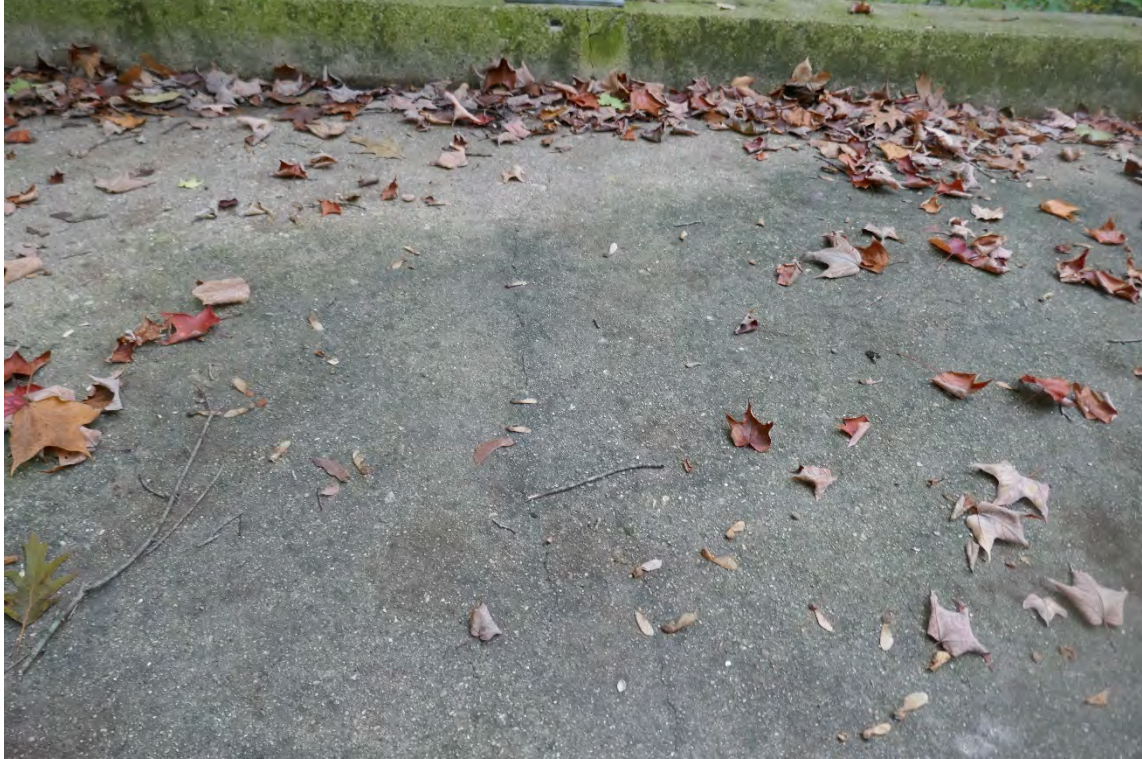
Transverse Cracking Noted in Top of Deck – 0.02” Max
